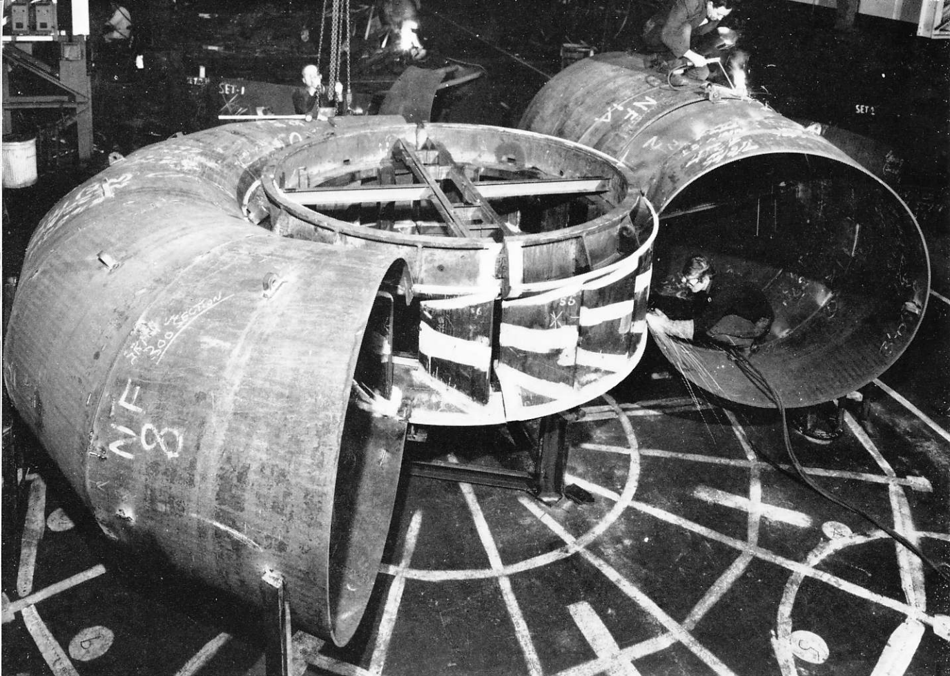
Welding up the spiral casing of one of the three 11,360 h.p. water turbines for the Nkula Falls hydro-electric project of the Malawi Electricity Supply Commission
