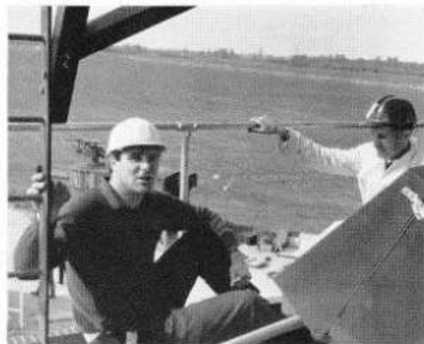
BELOW: Skid-lidded for safety, John Brand and John Chaplin take a breather in between jobs on the elevation platform. BOTTOM: An on-the-site conference for Ray Corduff, assistant site engineer, I. T. Butler, Apollo Project Manager, and Dick Muir
