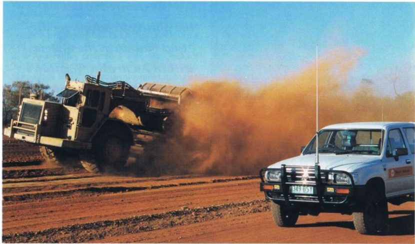
An armoury of equipment: An elevating scraper dwarfs a four-wheel drive while working on the RX access road
