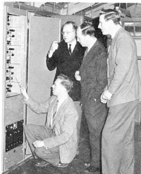
Left: Engineers examining part of the link transmitter equipment, from left to right, P. N. Sargeaunt, kneeling, of Baddow, H. P. Hall, D. A. Storrar and B. J. Clarke, of Radar Division
