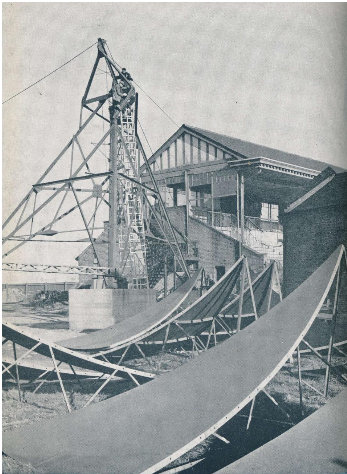
Cheeses for the dish. This is the preliminary stage of installation by Scanners at Galleywood of the thirty-foot dish aerial made at Newcastle. When it is complete, experiments on a forward scatter link between here and Start Point will begin. See the aerial being made on page 18
