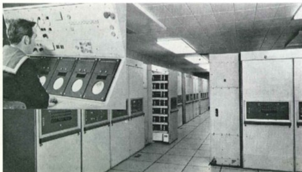
Marconi display back-up cubicles in the computer room at HMS Dryad with (inset) part of the Sea Dart radar operator's console
