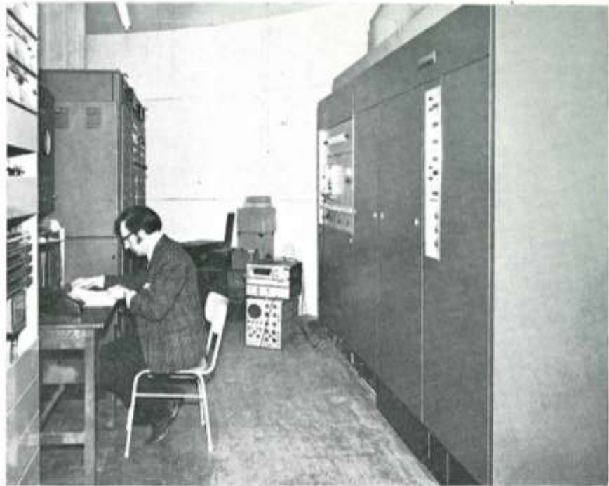
The new S2020 50cm transmitter/receiver installed at London Airport, as part of the nationwide improvements to Britain's air traffic control radar system being carried out by Marconi Radar Systems
