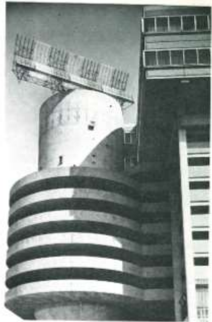
Rooftop aerial installation for a Marconi S650 radar, providing a 140-foot vantage point for Approach/Terminal Area cover at London's Heathrow Airport
